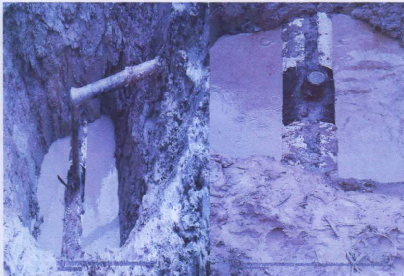
Figure 2: AFTER EXCAVATION 3" NIPPLE 3" BALL VALVE FOUND
